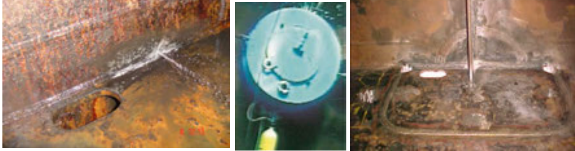
Plate and stiffener welded for crack repair with diving support through cofferdam installation
